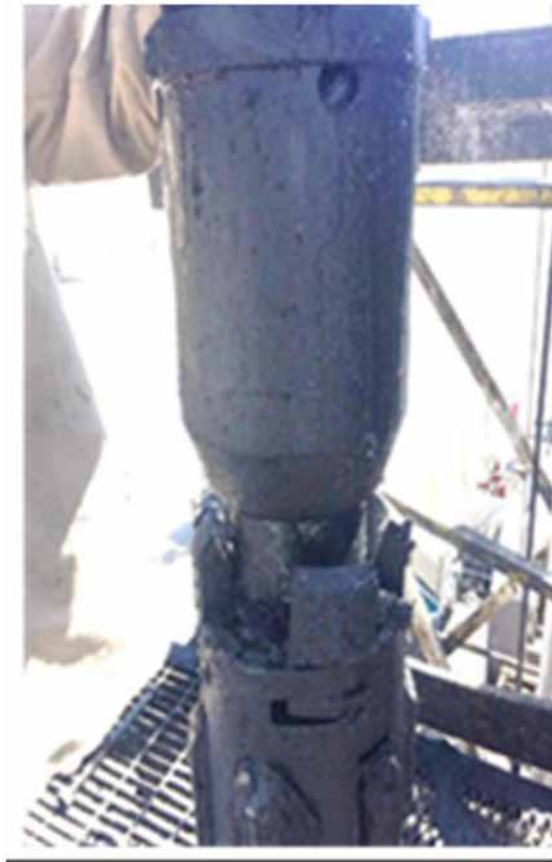
Figure 3—Well 58-32 packer damage
