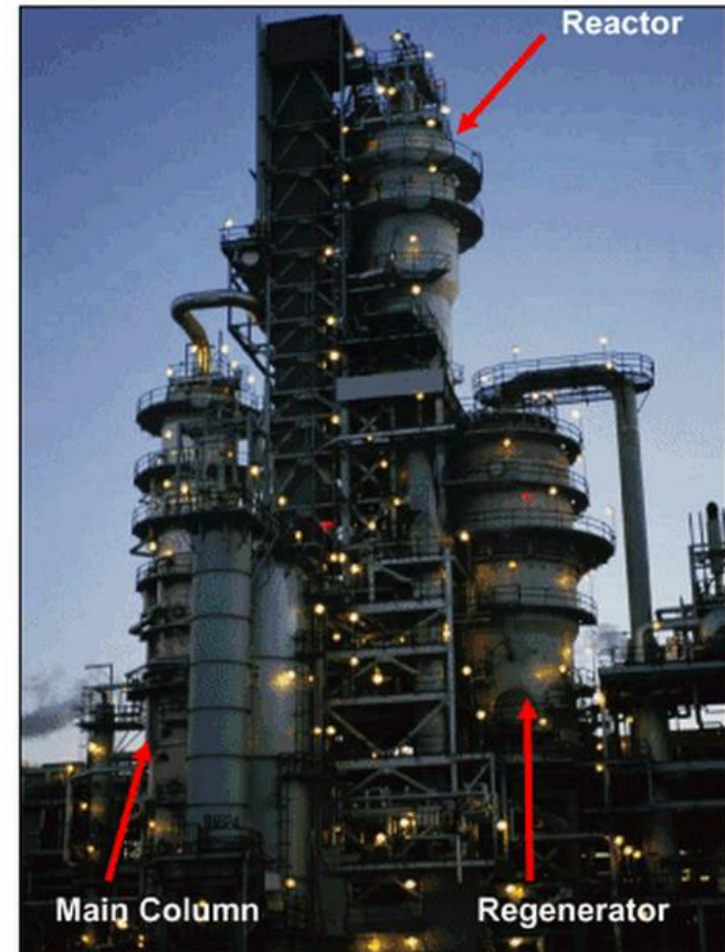
Fluidized Catalytic Cracker
