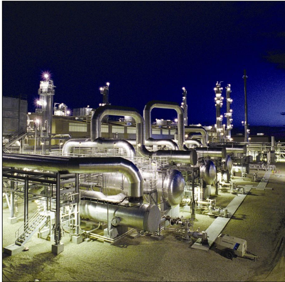
ConocoPhillips Lost Cabin Gas Plant
